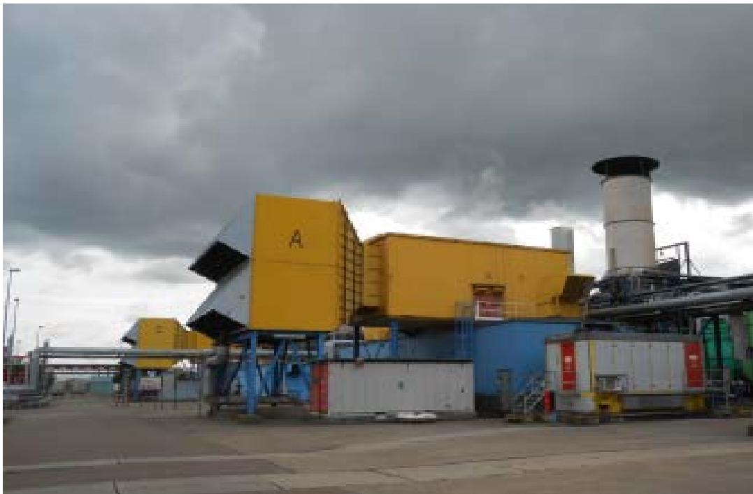
GT-A generating set with air intake filter and duct, stack, CO 2 -fire extinction container and electronic/electrical control cabinet
